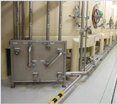
Piping system with fixed switching panels.
