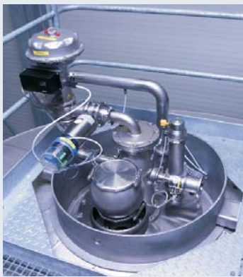
Tank connection in the tank top for CIP/Gas management
