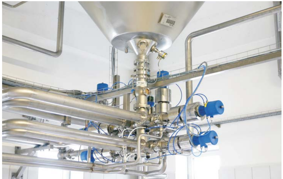
ECO-MATRIX tank connection in the new beer tower of Weißbierbrauerei Schneider, Kelheim
