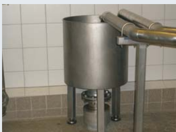
The drain construction with a layer of disinfectant liquid provides for an effective contamination barrier
