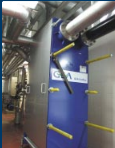
The heat exchanger used to elevate the wort temperature to almost boiling on its way from prerun tank to the copper.
