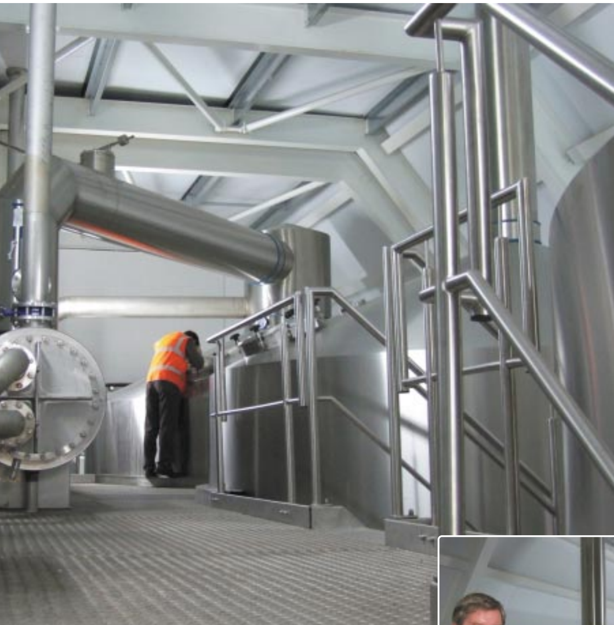
Adnams new Huppmann brewhouse showing the copper on the right connected to the vapour heat recovery cylinder on the left.
