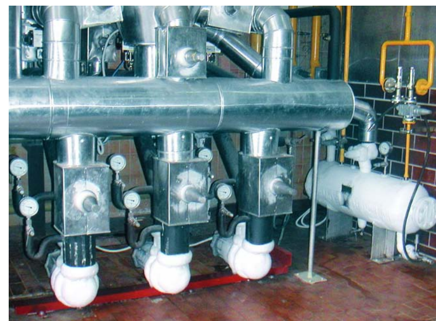
All refrigeration circuits have been fitted with new, maintenance-free ammonia pumps.
