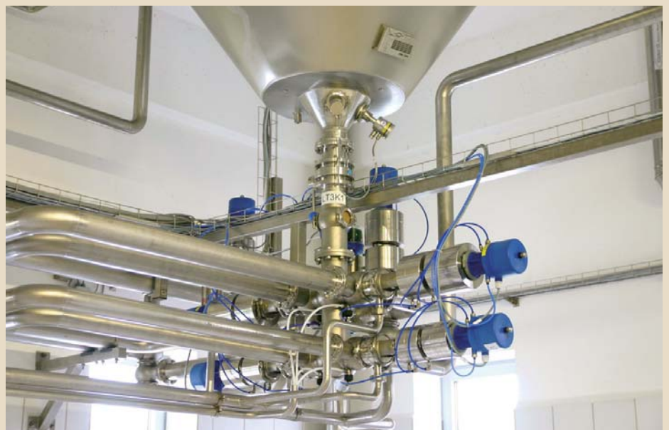
ECO-MATRIX® tank connection in the new beer tower of Weißbierbrauerei Schneider, Kelheim
