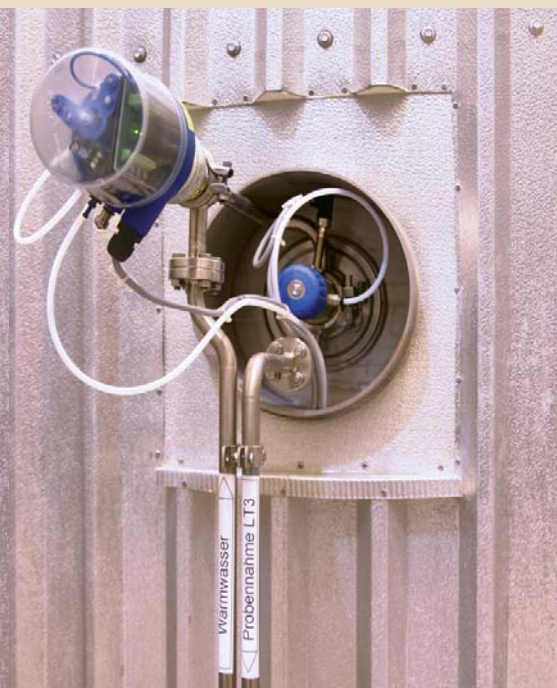
Sampling often involves the risk of contamination caused by unsterile piping. In the system at Weißbierbrauerei Schneider, cleaning and sterilisation is integrated in the piping and the process flow. The valves are installed flush with the tank, which allows optimal cleaning on the tank side
