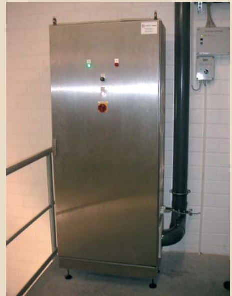
Fig. 4 Ionization system in the staircase
